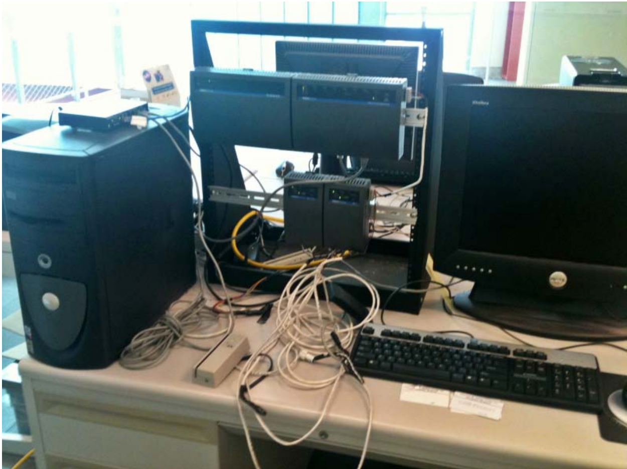
Figure 5.1: Building Automation System Test Bed
