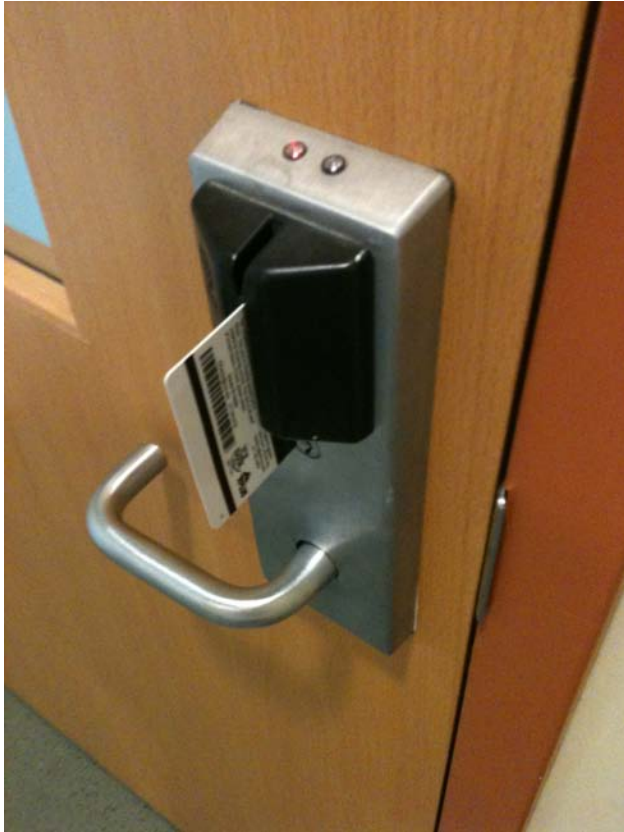
Figure 1.3: Swipe Card and Door Lock
